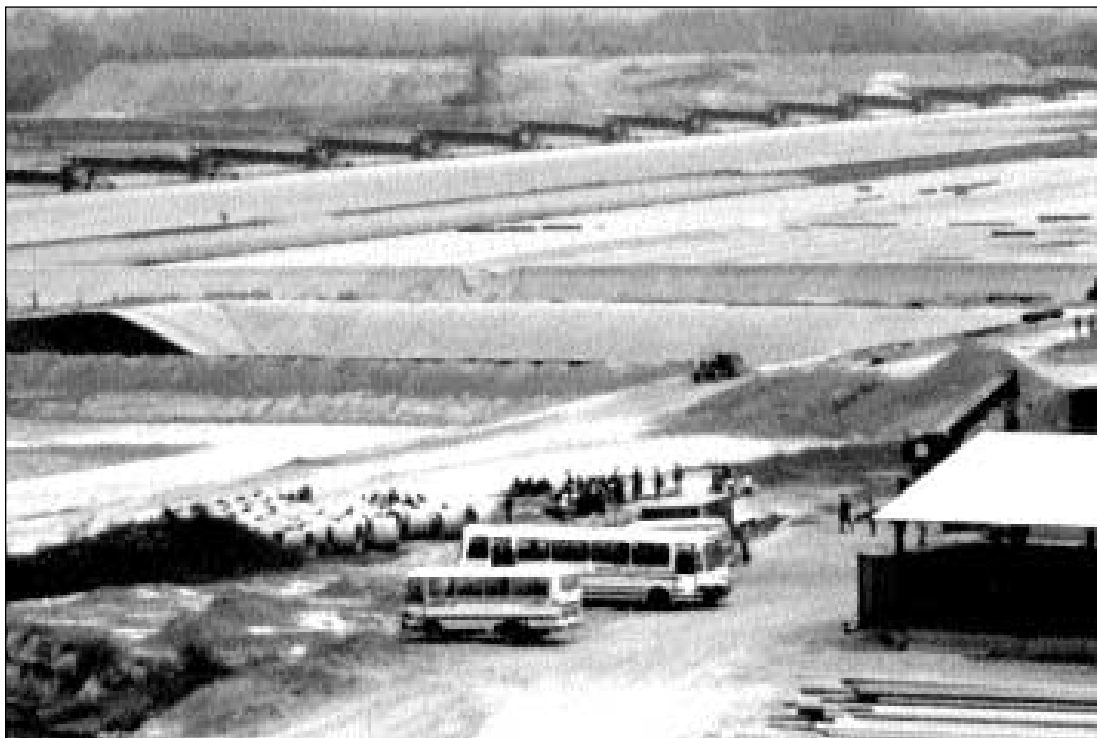
Lined pads being readied for cyanide heap leaching, Tarkwa gold mine, Ghana
